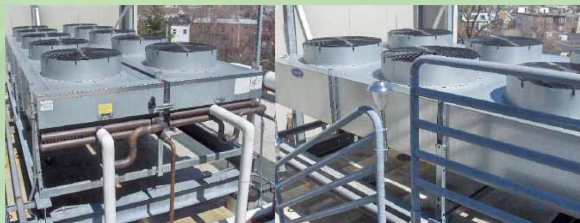
A new 115 Ton Air-Cooled Chiller located on the roof of the Cahill Building reduces the need for an oversized chiller and water tower operating during the winter months. Installation by MJ Flaherty
